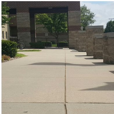
Image 24: Excessive Cross Slope in Walk
