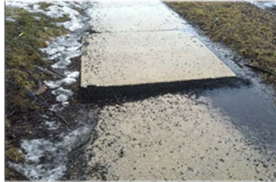
Settling and Ponding
