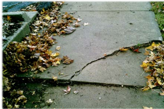
Defect with vertical faults
