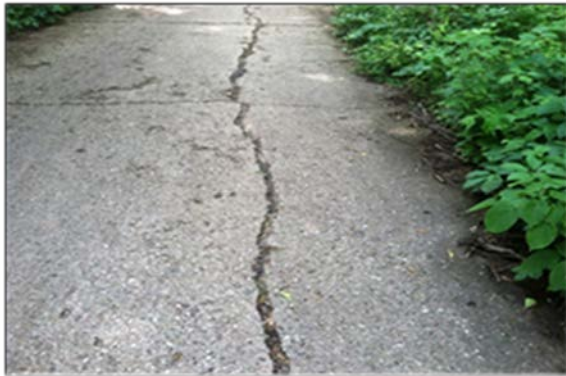
Settling and Cracking
