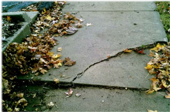
Cracking and Heaving
